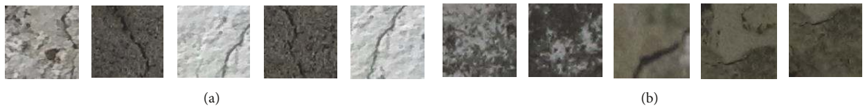
FIGURE 10: Illustrations of image samples containing anomalies: (a) cracks and (b) stains.
