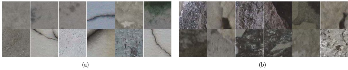
FIGURE 3: The collected image samples: (a) nonspalling class and (b) spalling class.
