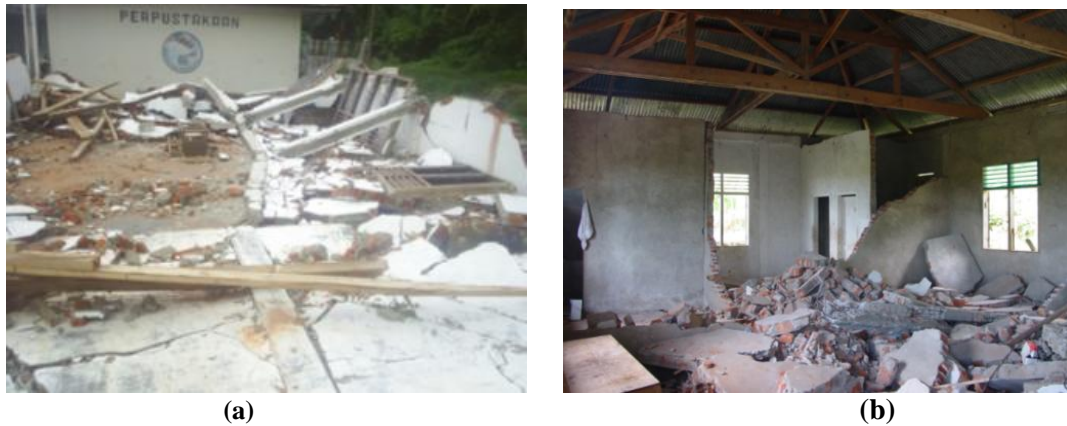
Figure 2. (a) A Totally Collapsed Reinforced Concrete Building, and (b) Collapsed Masonry Walls Inside a Modern Building.
