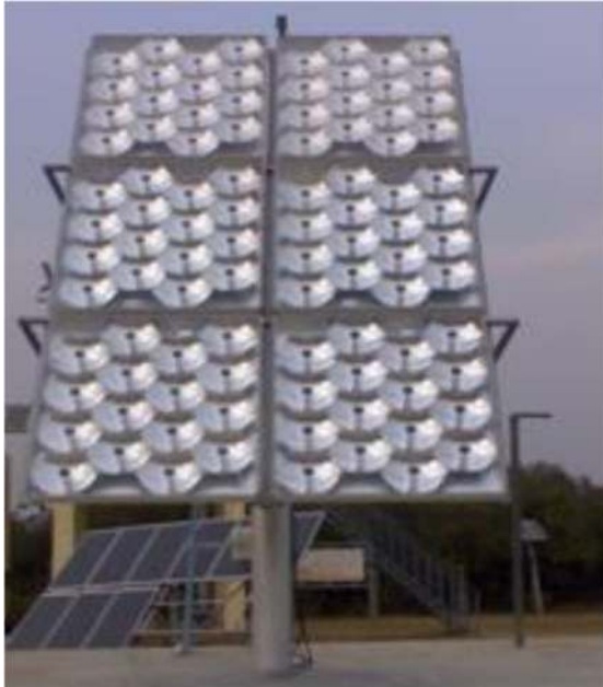
Figure 3. 1.2 KWp High Efficiency Solar Concentrator with Tracker being installed at IIT Kanpur Courtesy: Moser Baer Photovoltaic Pvt Ltd.
