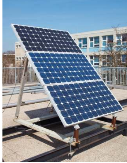
FIGURE 1: Our PV system used for data monitoring during the solar eclipse.
