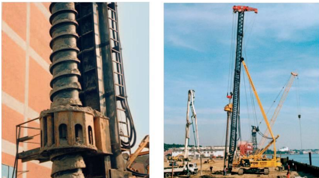
Figure 9 – VB auger with large hollow stem (left) and VB piling rig (right)
