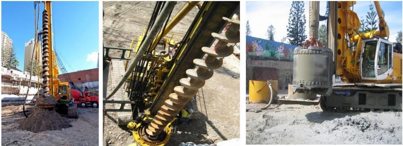
Figure 7 – Screw piling application using CFA augers (left and centre) and a conventional rotary bored piling application (right)
