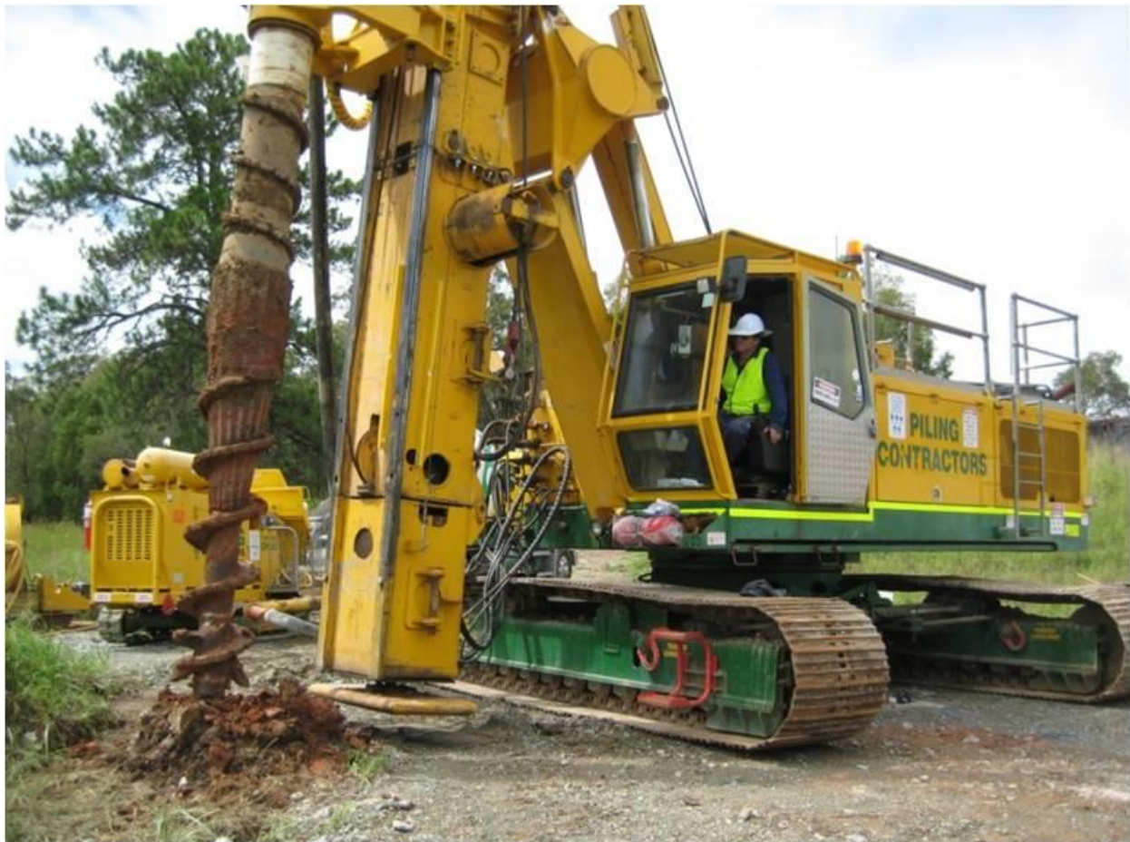
Figure 88 – Installation of test piles B, C and D with the Casagrande C30 piling rig
