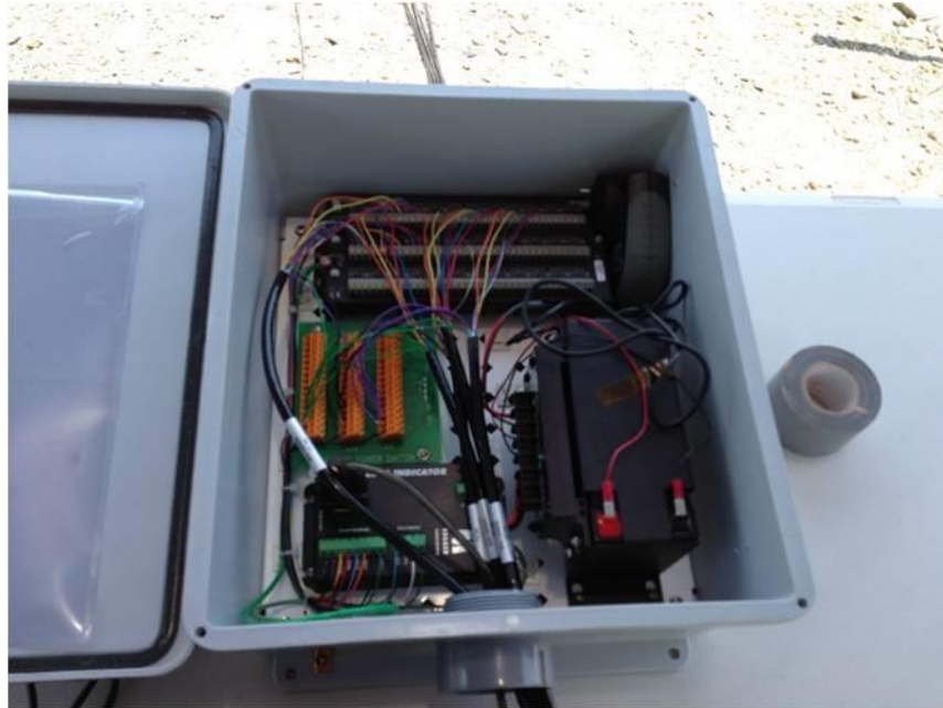
Figure 59 – Data readout unit used for the tests at Lawnton
