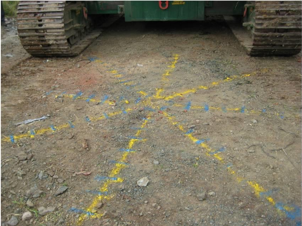
Figure 64 – Survey points for the determination of vertical soil movements during pile installation at four different axes for test pile E
