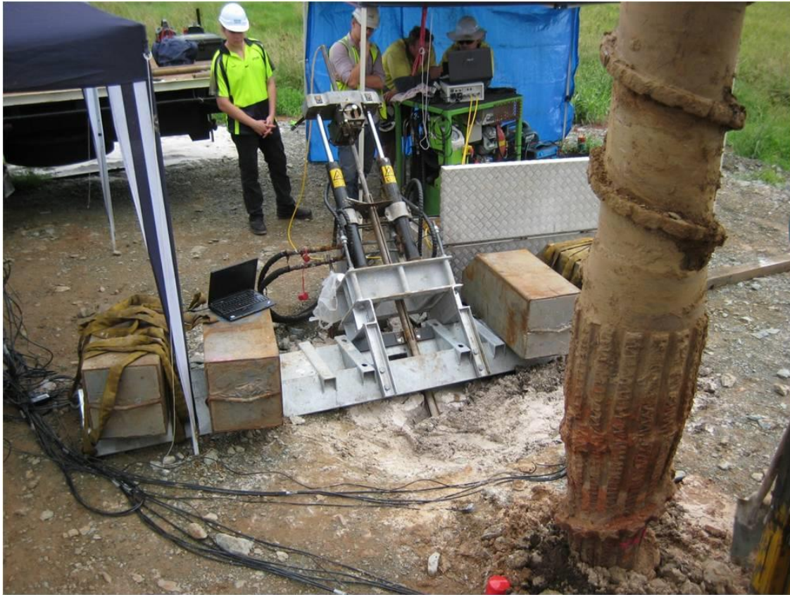
Figure 57 – Raked CPT setup on site during the installation of a test pile (Pile C)
