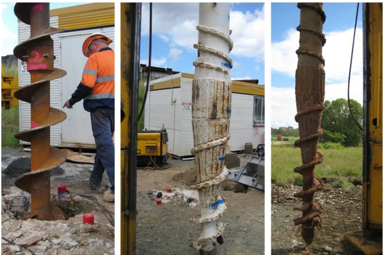
Figure 86 – The three different augers on the field test site, CFA (left), progressive displacement (centre) and rapid displacement (right)
