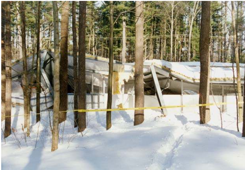
Figure C8. Collapsed Jackson Landing Skating Rink
