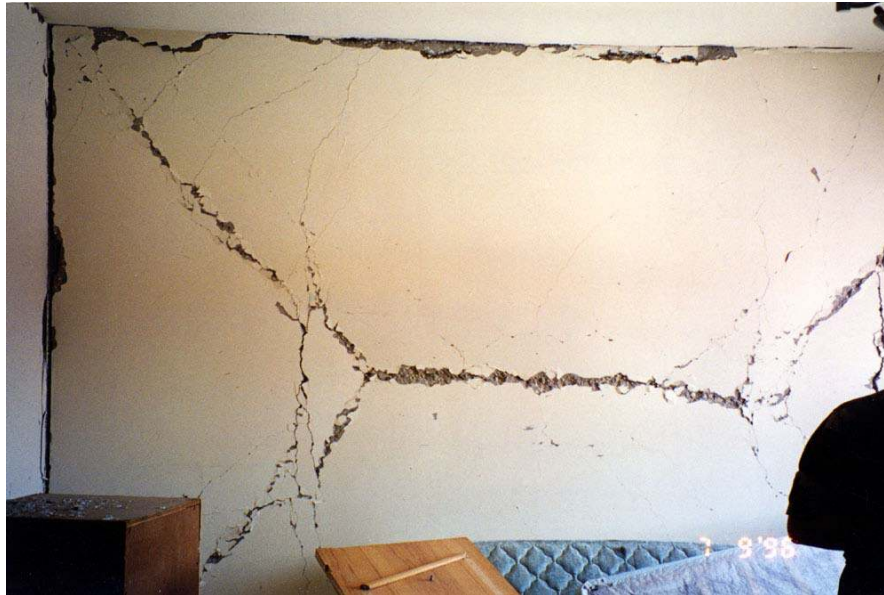
Figure C22. Interior wall exhibiting yield line damage
