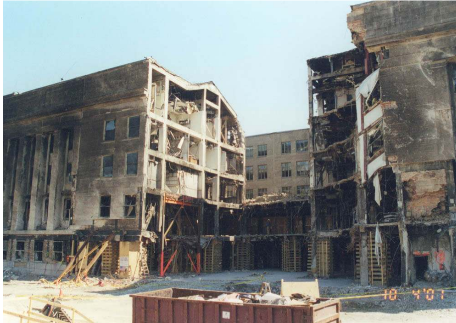
Figure C14. Collapse area after debris removal
