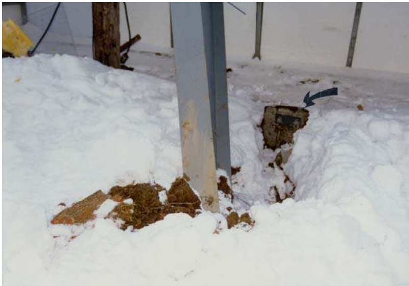
Figure C11. Split pier (arrow) at failure initiation location
