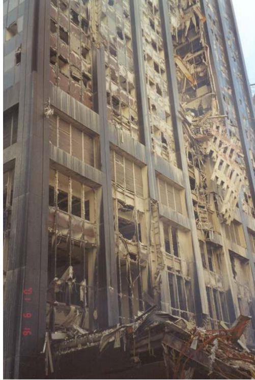
Figure C16. Gash in North Face of 130 Liberty Street
