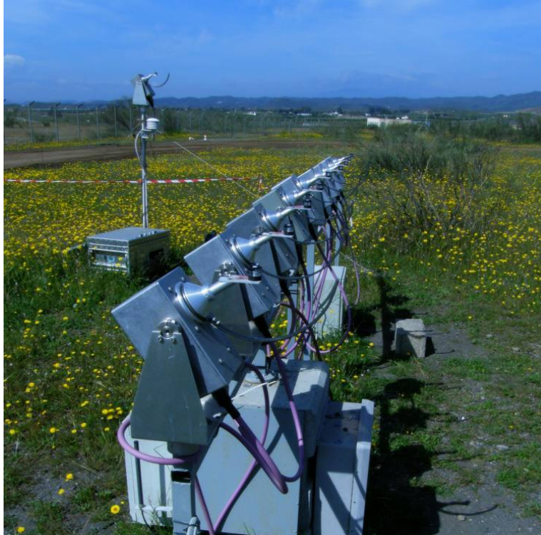
Figure 3-17. RSI calibration station at Plataforma Solar de Almería. Photo from Stefan Wilbert, DLR
