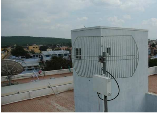
Figure 6: One example situation where the Theni to Vijerani link was completely obstructed by newly constructed elevator shaft. This problem was not resolved until we visited Theni after 2 months.
