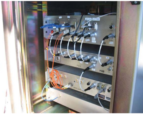
Figure 5. The RF-shielded rack housing BIGHORNS back-end components (from the bottom to top : box with a second gain stage and RF-filters; BEDLAM spectrometer; power unit; and PC computer unit).
