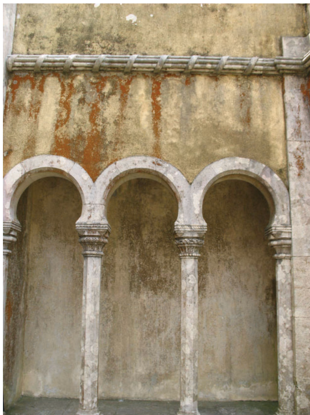
Fig. 1. Wall of the Palácio Nacional da Pena, Sintra (Portugal), showing extended colonization by Trentepohlia sp.
