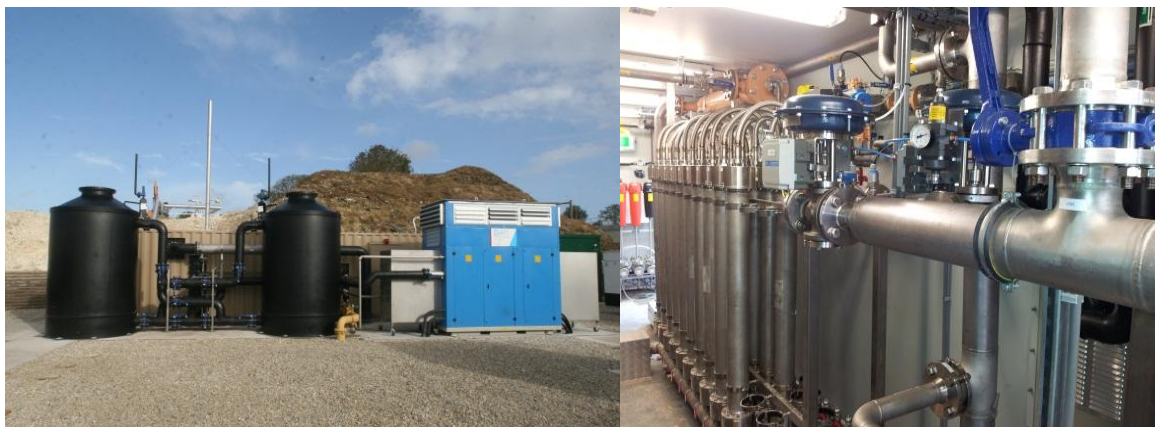
Figure 16 The membrane biogas upgrading plant in Poundbury with a capacity of 650 Nm 3 /h raw biogas. Images from DMT.
