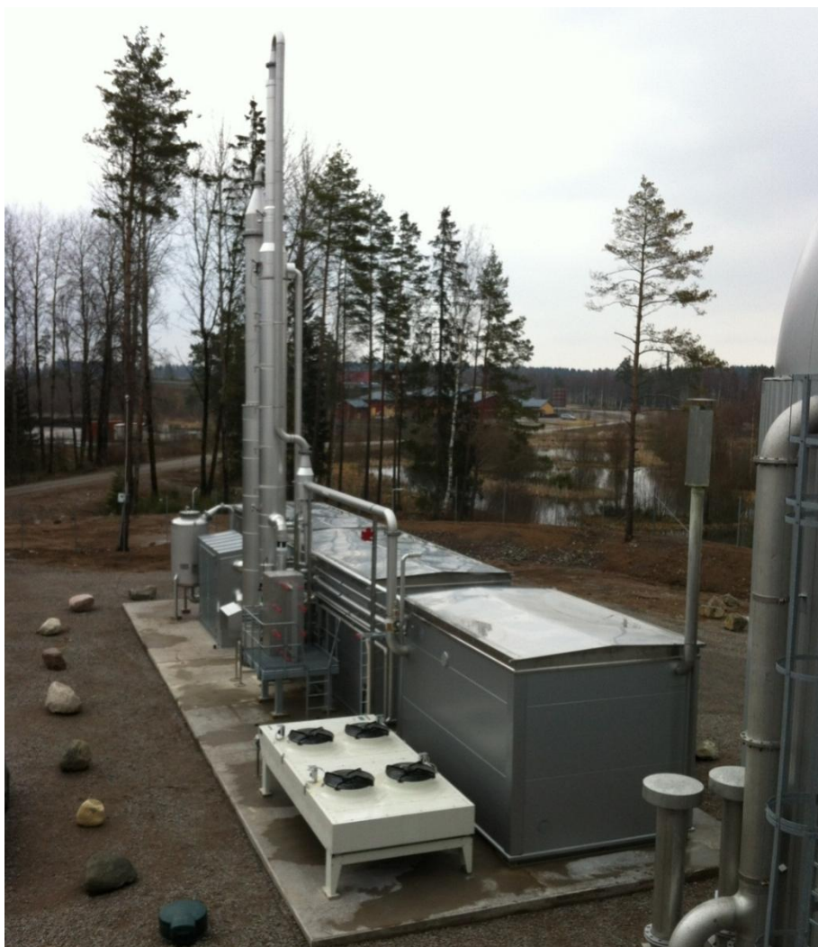
Figure 4 An amine scrubber used for biogas upgrading in Sweden. Image from Purac Puregas.
