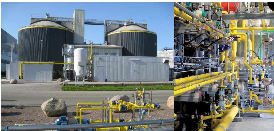
Figure 8 PSA upgrading unit in Sweden. The exterior view (left) shows, from the left, the catalytic oxidizer, active carbon filters, pressure levelization tank (white) and a container with the PSA columns. The interior view (right) shows valves and PSA columns. Images from E.ON Gas Sweden.
