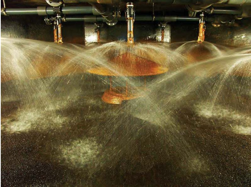
Figure 2: Full-scale trickling filter at Oasen WTP Lekkerkerk. Raw water is sprayed directly on top of the filter bed. The central outlet with cone is used for drainage of backwash water.
