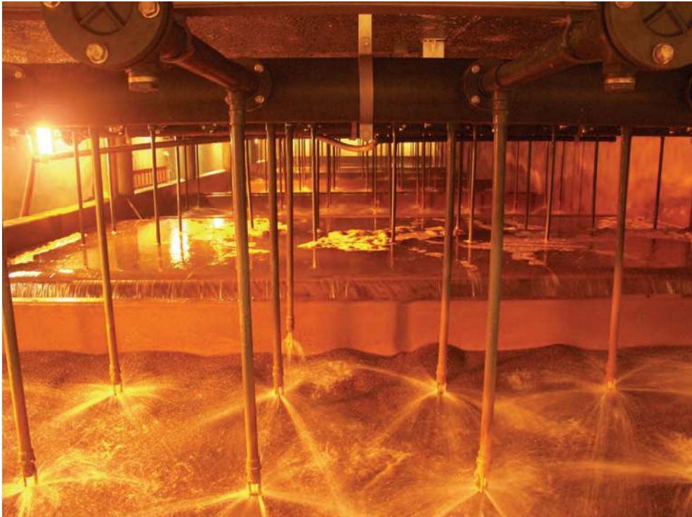
Figure 2: Oasen DW trickling filters in production (front) and during backwash (background)
