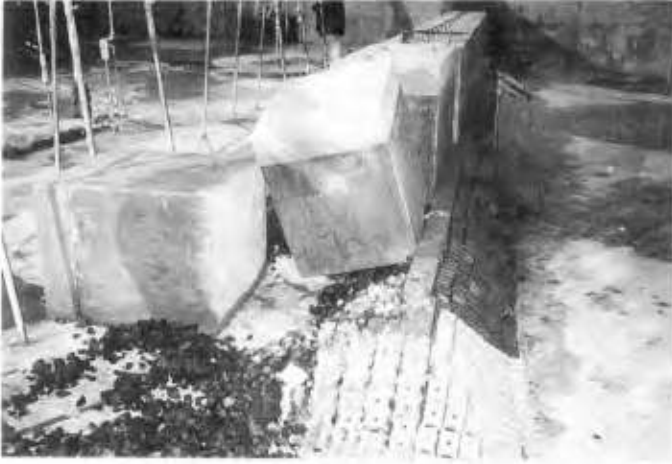
Photo 1. Damaged Caisson and Mound of the Outer East Breakwater
