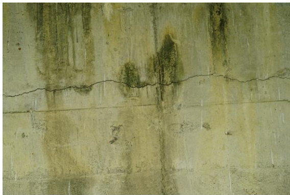
Figure 15. Crack image case 2
