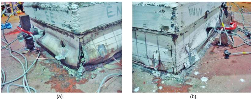
Fig. 10. (a) Damage at east column at 3.62% drift; (b) damage at west column at 4.35% drift
