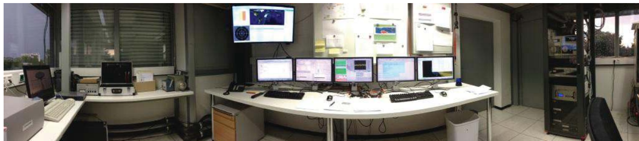
Fig. 12.— Control room for the ground station at Graz University of Technology
