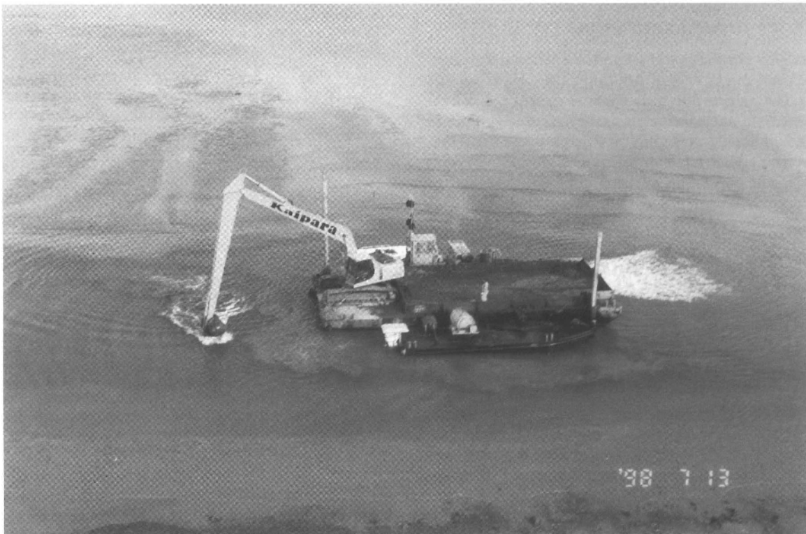
Figure 3. The dredging of muddy sediments from the marina approach channel using a digger mounted on a barge.
