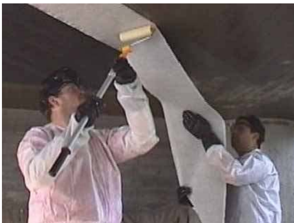
Figure 4-3: Hand lay-up. The light colour shows paper to be removed, Täljsten and Carolin (1999)
