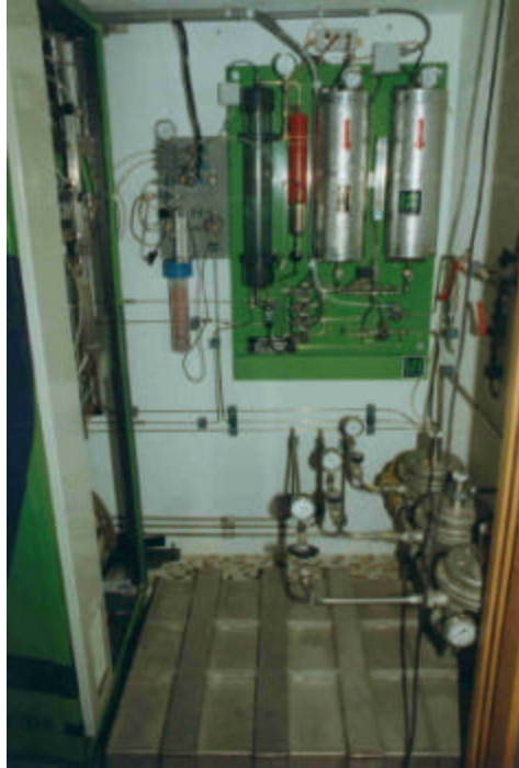
Picture 2.4: Purification unit (on wall) and metal hydride storage tank (on ground).
