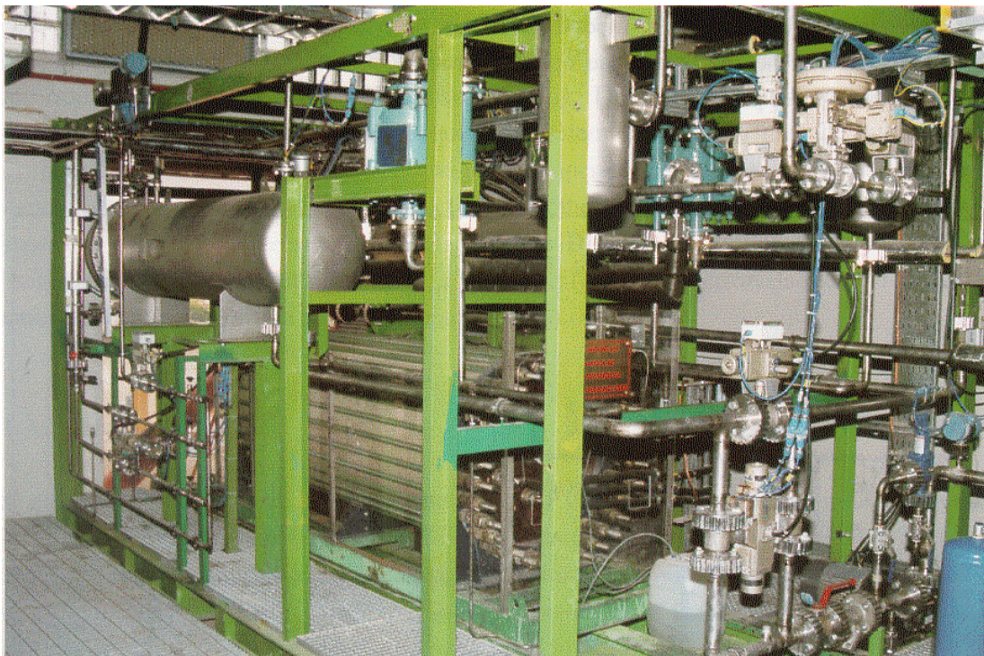
Picture 11.2: HYSOLAR Process Room with 350 kW Electrolyzer in Riyadh
