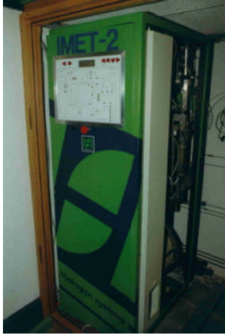
Picture 2.3: Electrolyzer and regulation display
