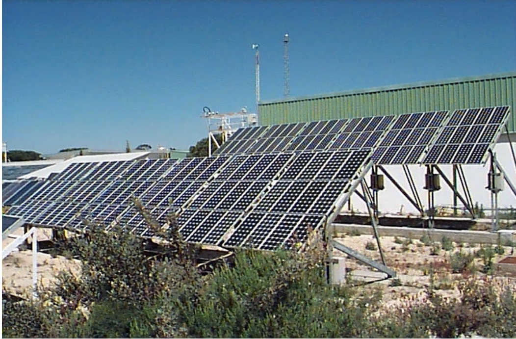
Picture 6.1: Photovoltaic field
