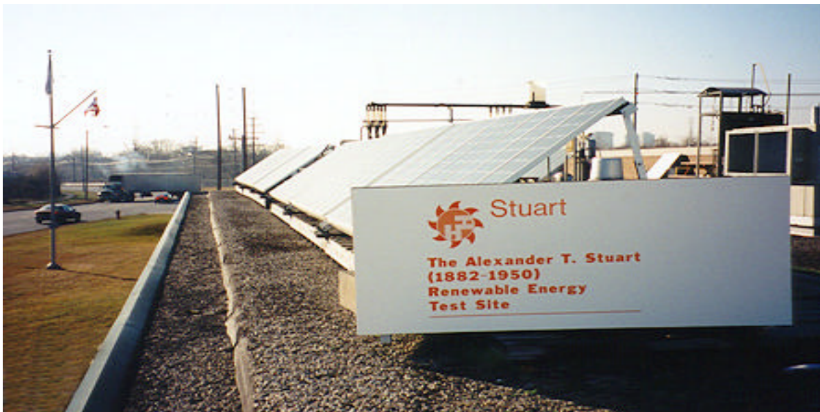
Picture 3.1: Photovoltaic Array of the Renewable Energy Test Site
