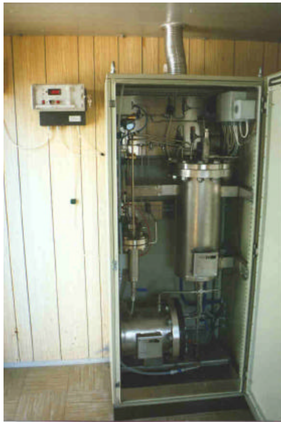
Picture 9.2: The 2.25 kW electrolyzer
