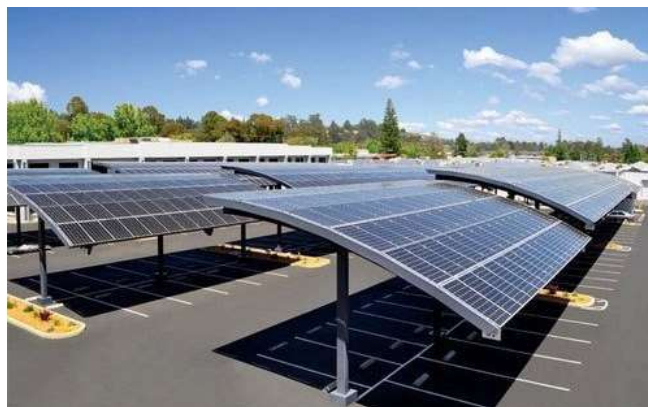
Fig. 2. Example of carport with integrated PV system.
