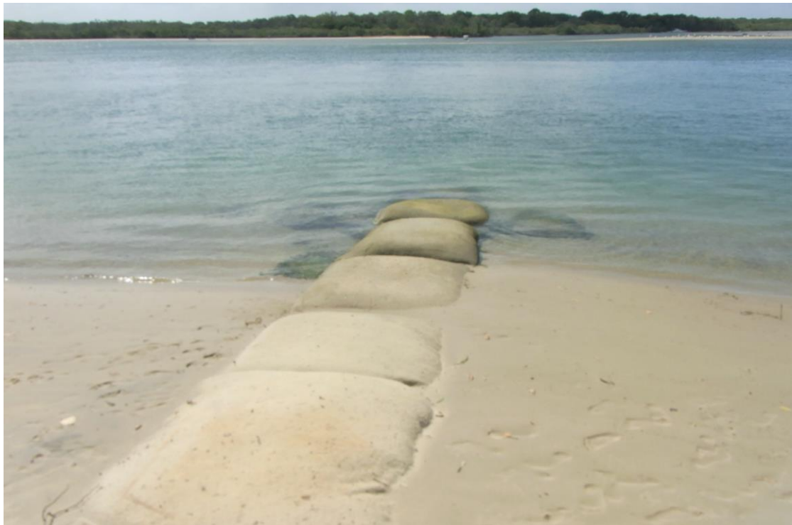
Figure 12. Photos showing up to 2m change in beach width and up to 0.2m change in beach height at Groyne
