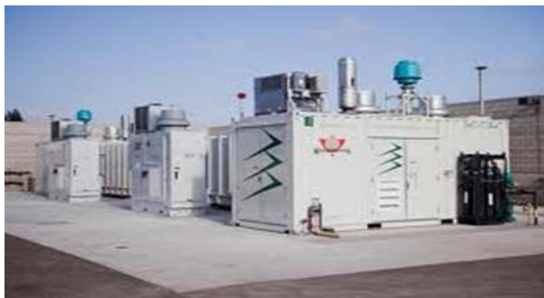
Figure 6-1. Commercial Fuel Cell for CHP Application
