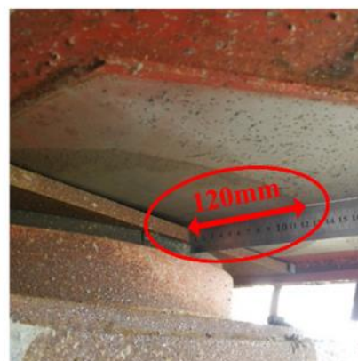
Support slipping on Pier P33
