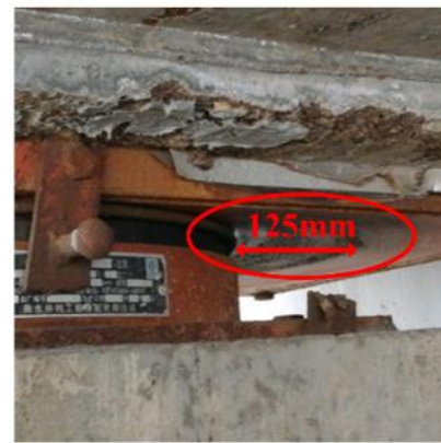
Support slipping on Pier P30
