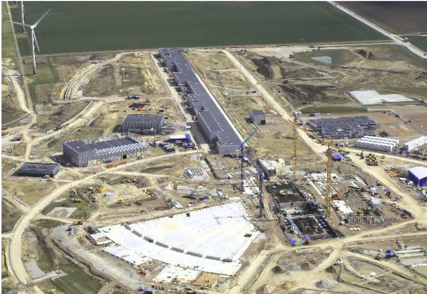
Figure 11.1 The construction site of the European Spallation Source on 2017-04-17. The long gray building is the RF gallery that will house the RF systems of the ESS accelerator. Photo credit: ESS.
