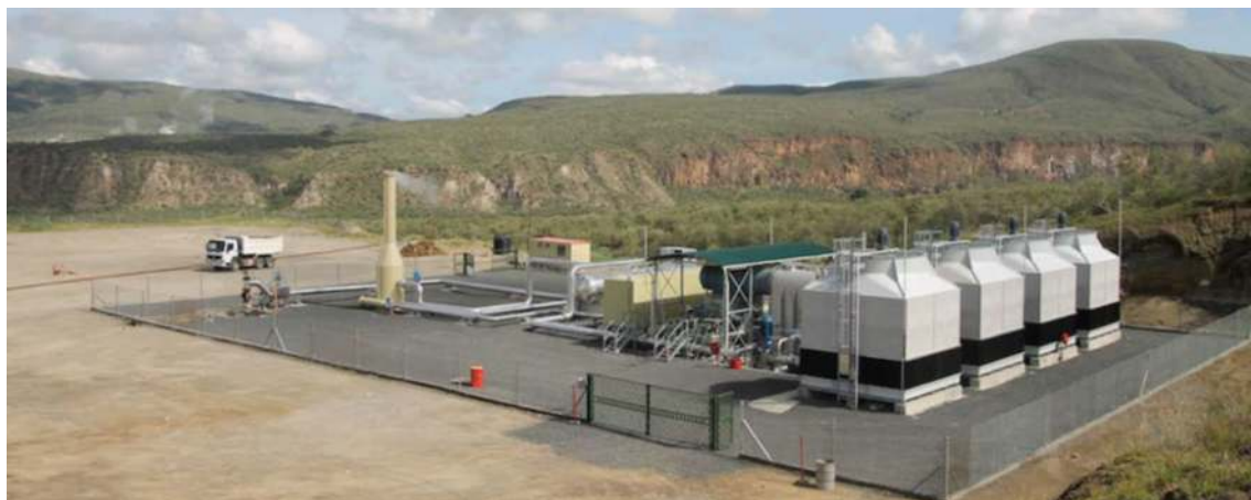
Fig. 5 A GEG 5-MW C50 wellhead plant at Olkaria in Kenya [53]
