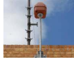
(c) Installed antenna node
