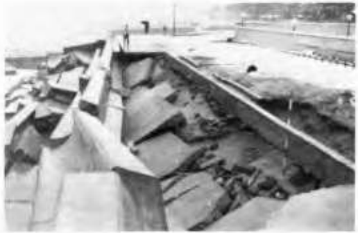
Fig.10 In January 1961, the stepped face seawall had been partly destroyed by the winter strong wave force. Waves had scoured beach at the foot of the seawall, and the body of the seawall had been scattered. The seawall had been reconstructed at once.
