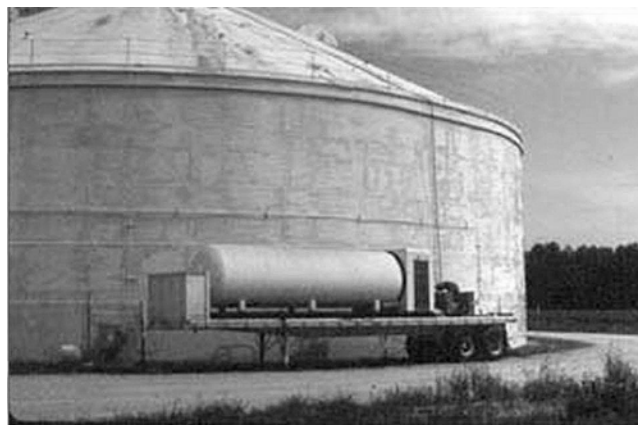
Fig. 1. Application of carbon-dioxide-based modified atmosphere in a large silo bin in Kingston, NC, U.S.A.
