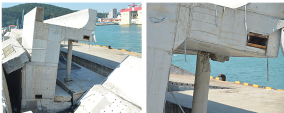
Fig. 1. Destruction of the upper structure of Gamcheon Port breakwater by typhoon.
