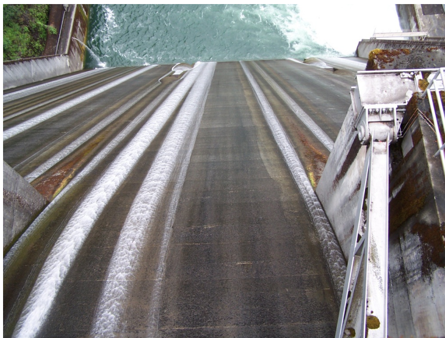
Figure 4.1. Spillbay 3 at Detroit Dam showing the rough, irregular concrete surface.
