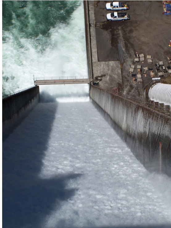
Figure 4.2. Spillbay 6, 3.5-ft gate opening (3090 cfs), showing walls confining the turbulent flow created on the rough spillway chute.
