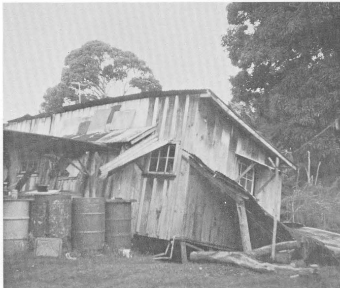
FIGURE 40.—January 13, 1960. House built directly over the Kapoho fault scarp tilts backward (north) into the graben. Photograph by Howard Pierce, Hilo, Hawaii.
