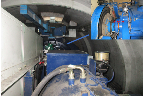
Fig. 3: Panoramic view of wind turbine nacelle and horizontally installed sensor.
