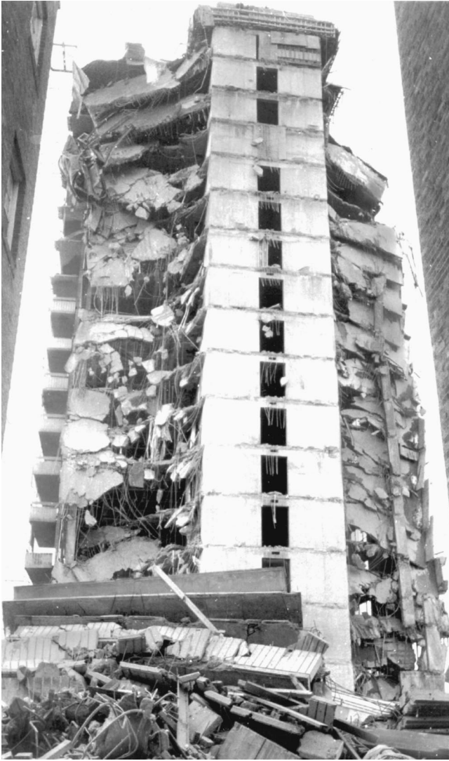
Fig. 2. Building collapse; four men missing and three injured when apartment under construction collapsed in Brighton [from Boston Globe , January 26, 1971; republished with permission]
