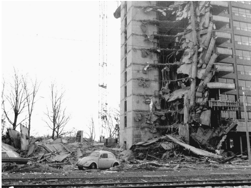
Fig. 1. Chunks of concrete and wood were strewn across MBTA track (in foreground) by building collapse [from Boston Globe , January 26, 1971; republished with permission]
