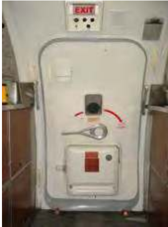
Figure 99. Examples of emergency exit locking mechanism marking and emergency exit locator sign in passenger aircraft.
