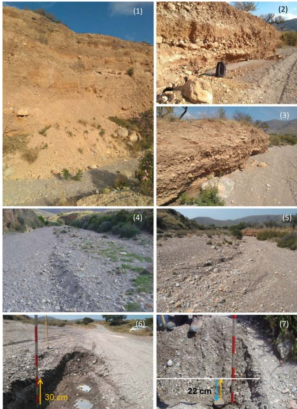
Figure 12. Local material collapses in composite detrital banks after basal undermining caused by the flash flood of April 2019 (1,2); entrainment and surface washing of non-cohesive basal bank deposits during the peak flow of September 2019 (3); after the larger event, greater morphological adjustments occurred: lateral accretion of central longitudinal bars in the Upper RCR (4), vertical accretion at the head of a central bar and slight incision on the thalweg bed in MDR (5), a strong net deposition between the upper and Middle RCR (see the levellogger plate that was deeply buried) (6), and high transitory erosion in the main active channel (see a clear example in the Upper RCR) (7).
