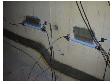
Fig. 7. View of typical strain gage configuration mounted on the bridge itself (lower left: Fig. 6).
