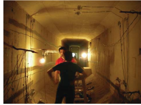
Fig. 6. View inside the box girder showing the scale and the environment in which the sensors are mounted.
