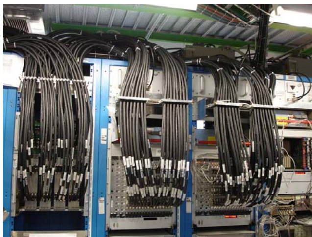
Fig. 4. One quarter of the analogue cable inputs into the preprocessor system. Supporting stocks are located at about 2/3 of cable height
