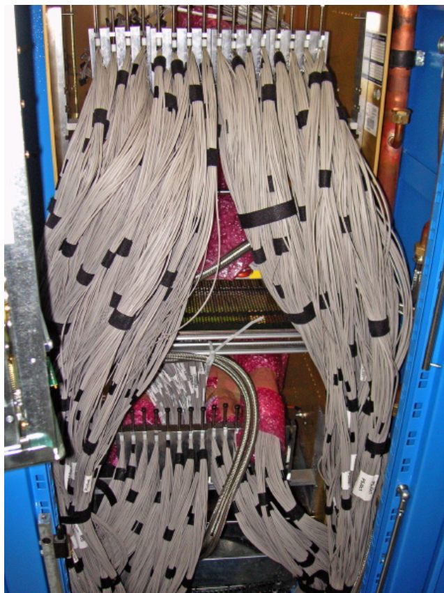
Fig. 5. Full LVDS input cabling at the back of a JEP crate
