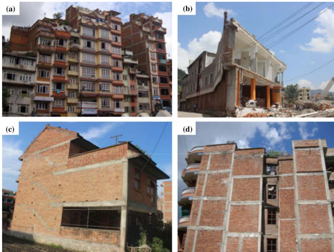
Fig. 5 a A neighborhood in Kathmandu metropolitan city with dominance of slender structures. b Asymmetric building with severe damage in Kathmandu. c Columns too less and not even in grid.
