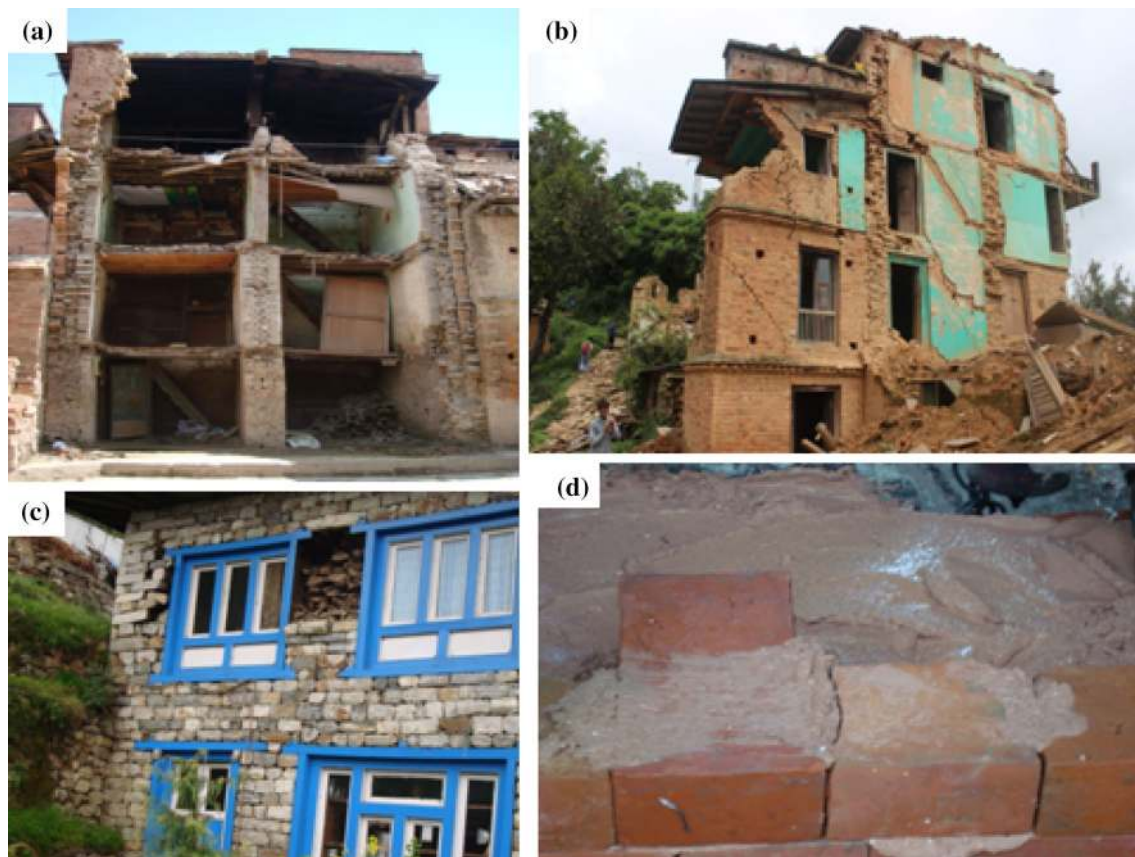
Fig. 10 a Out of plane collapse of load bearing masonry wall in Bhaktapur. b Heavily damaged masonry structure in Chautara due to out of plane collapse of majority of walls. c Delamination of wythes
