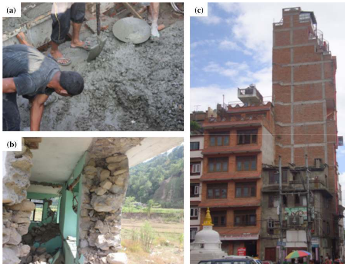
Fig. 4 a Common concrete mixing method with high water cement ratio in residential constructions. b Damaged wall due to improper binding on rounded aggregates in Melamchi (Sindhupalchowk). c An example of slender structure in Kathmandu metropolitan city
