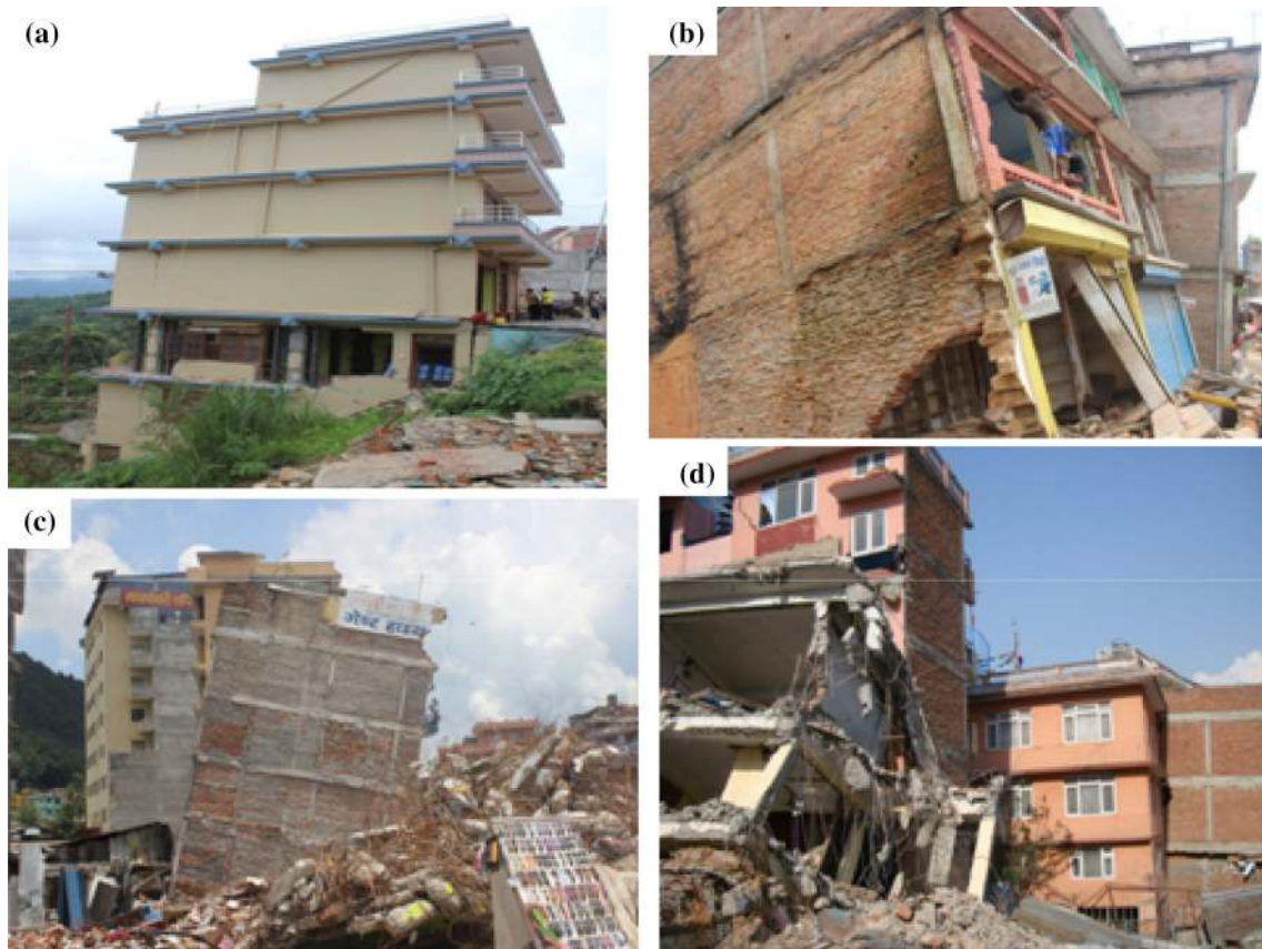
Fig. 9 a RC building in stepped foundation with partial damage. b Building tilted with column failure due to stepped foundation. c Large displacement in foundation led tilting of building constructed
