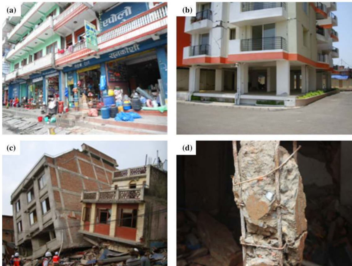
Fig. 1 a Ground floor of residential buildings without infill walls. b Ground floor of an apartment building without infill wall. c Soft storey and structural pounding failure. d 16 mm diameter rebar but only four in number (corroded as well) from a collapsed building in Kathmandu
