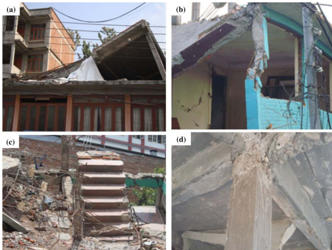
Fig. 2 a Collapsed column due to welded vertical re-bars. b Column failure due to large gap of stirrups. c Outwardly placed 6 mm diameter re-bars exposed on collapsed structures. d Poor beam column connection with exposed re-bars
