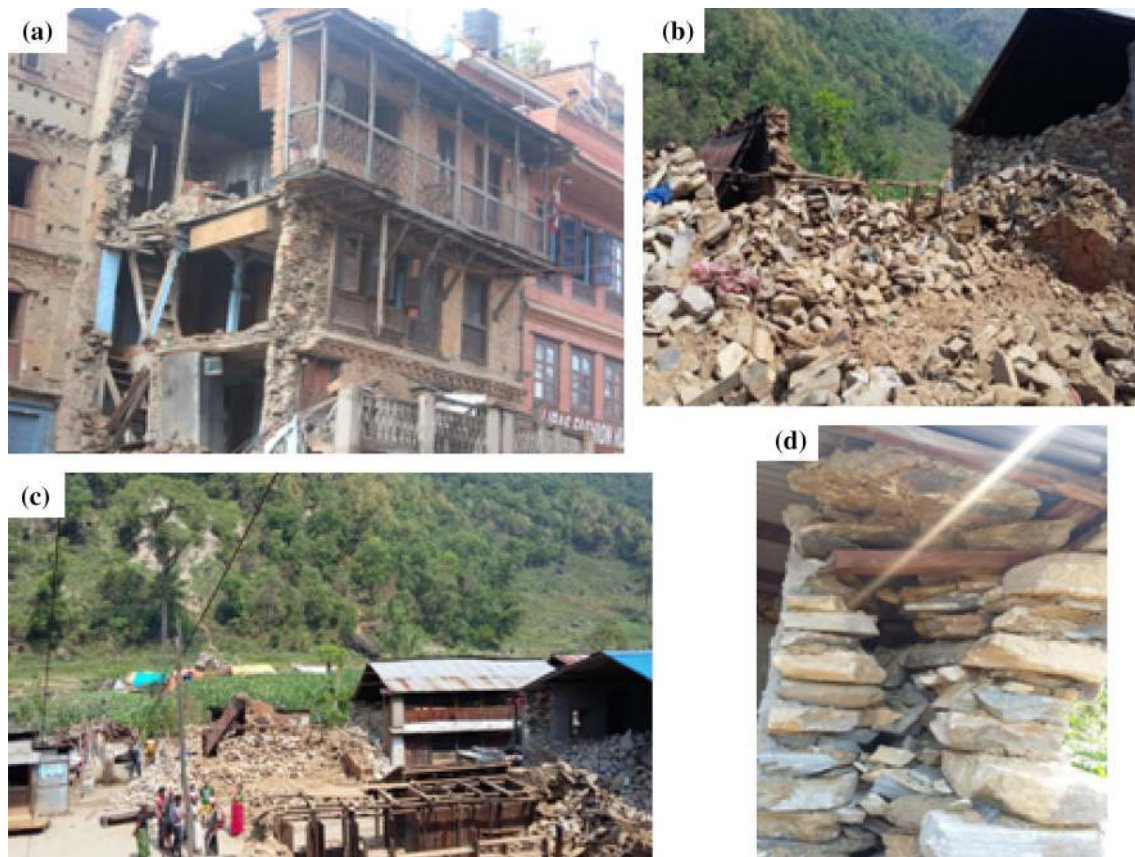
Fig. 15 a Pounding and progressive failure on the building situated on edge. b Complete collapse of row houses in Baluwa (near epicenter). c Progressive failure on row houses and good performance of timber frames. d Separated wall due to structural pounding
