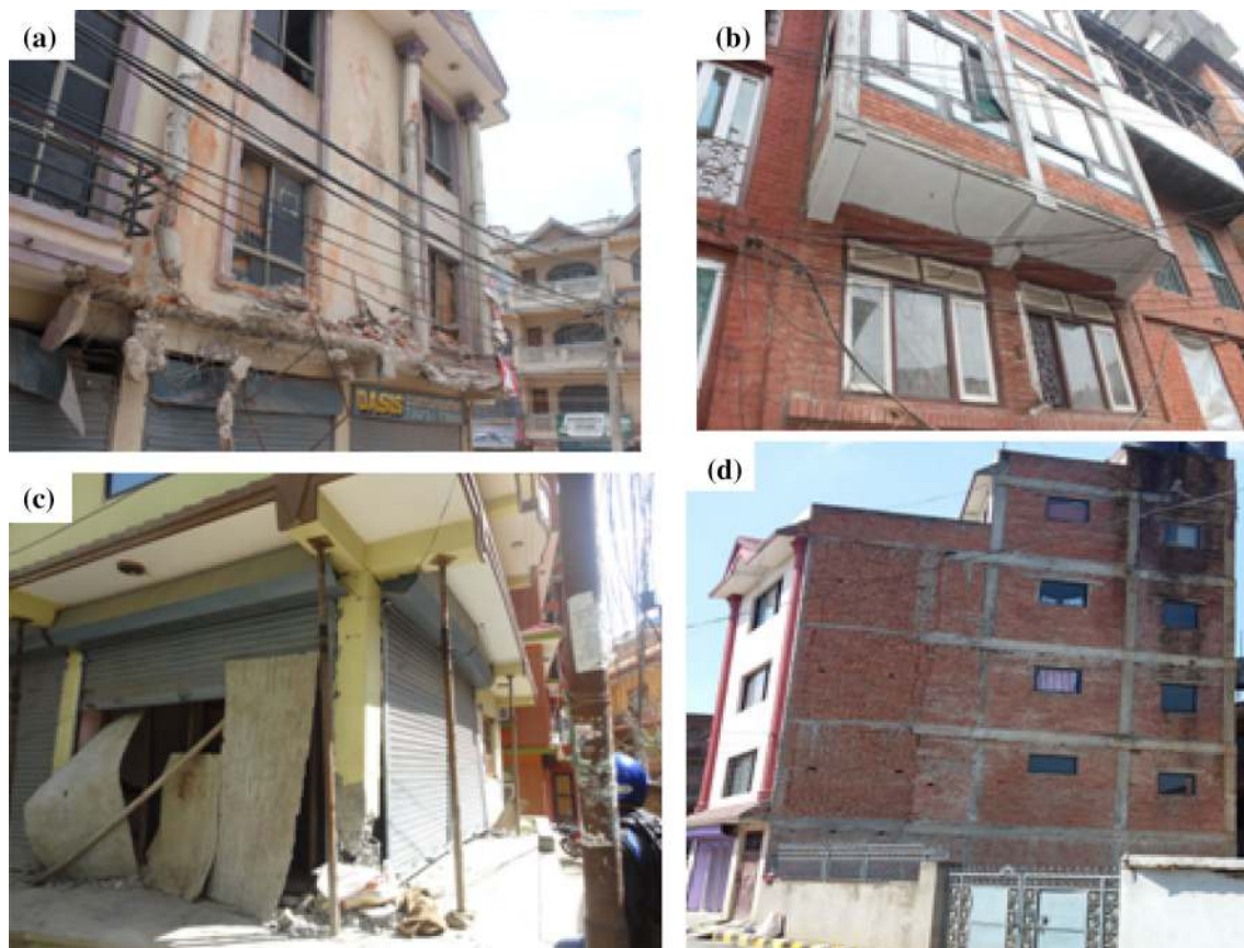
Fig. 3 a Floating column with projected construction in upper stories. b Floating columns and continued construction in upper stories. c Column buckling in a building with cantilevered construction and floating column. d Large cantilevered construction projected from structural system
