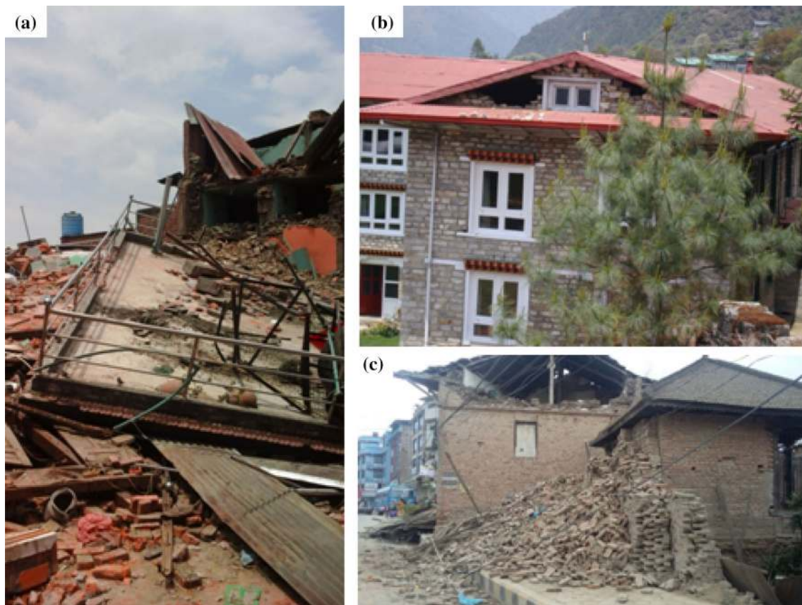
Fig. 14 a Complete collapse of RC slab used as roofing in a masonry building. b Out of plane failure of gable portion of a stone masonry building. c Heavy gable portion out of plane failure in brick masonry
