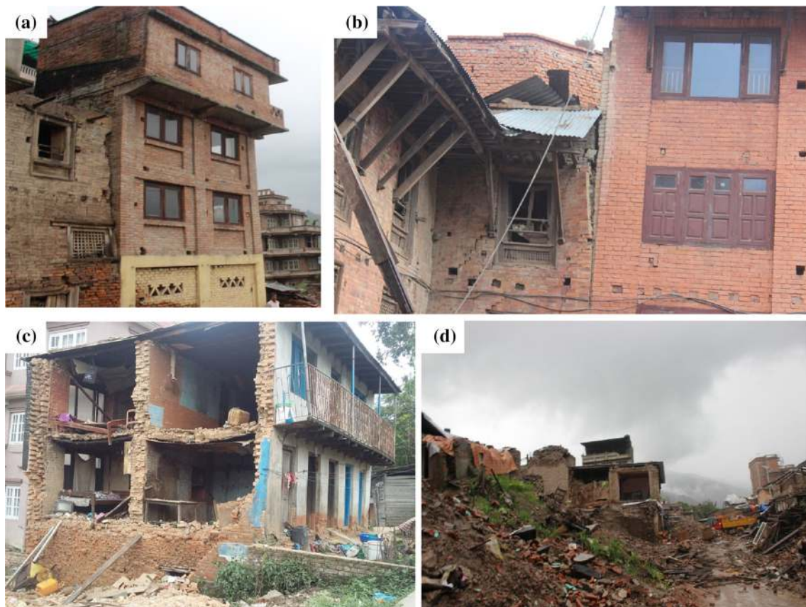
Fig. 12 a Heavy load concentration in the fourth storey of a masonry building. b Re-entrant corner and associated damage in masonry building in Bhaktapur. c Lack of connection led collapse of wall. d Heavy damage in old masonry houses in Sankhu
