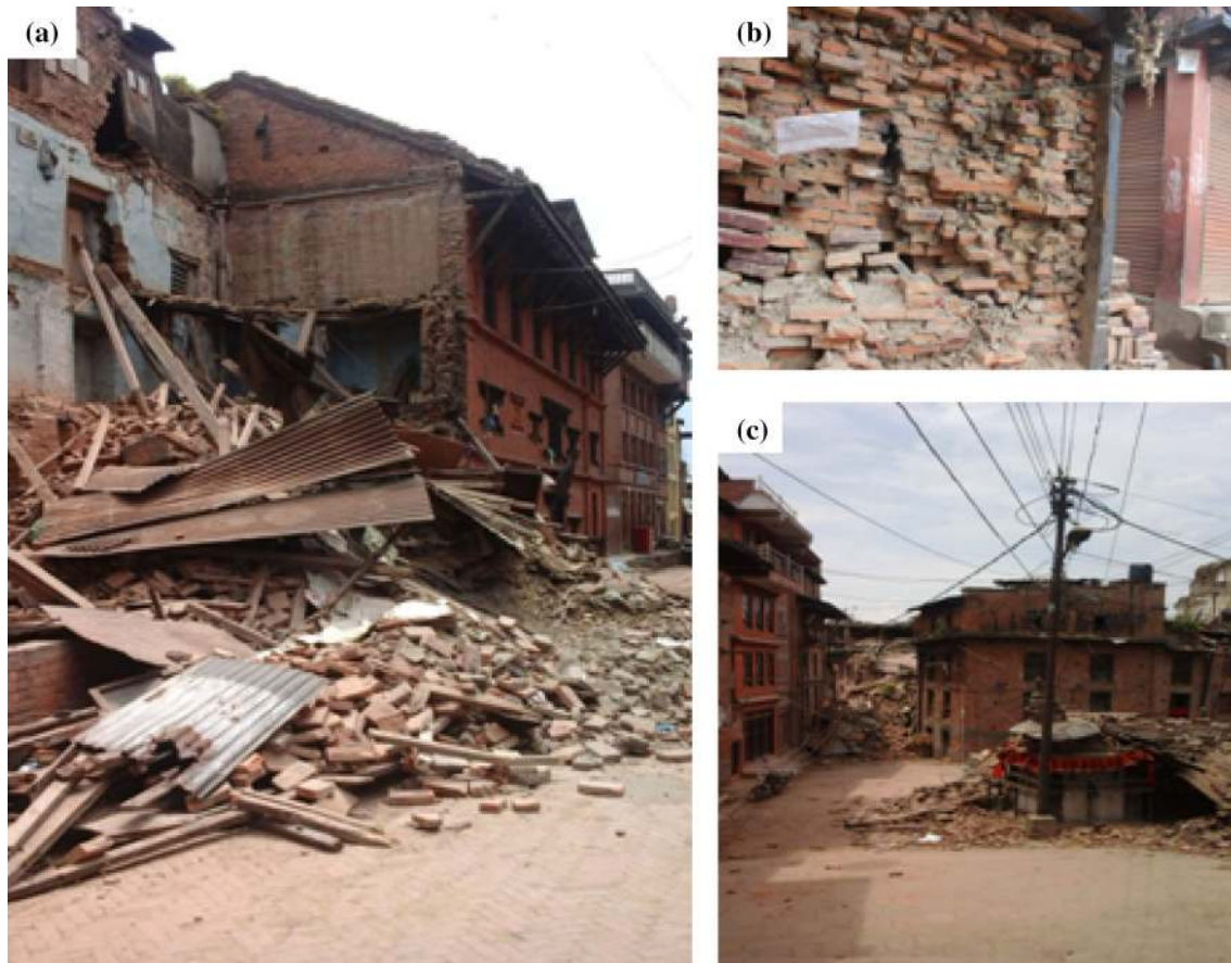
Fig. 13 a Damage in shared wall. b Segregated mud mortar and associated delamination of wythes. c Damaged building with inclined foundation and intact buildings having leveled foundation
