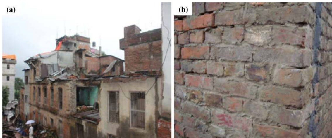
Fig. 11 a Failure of masonry units due to lack of proper binding. b Mud mortar used for reconstruction of URM building destroyed during 2015 Gorkha earthquake at Bhaktapur
