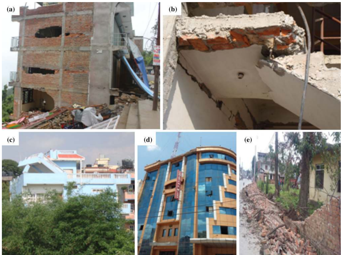
Fig. 8 a Out of plane collapse of brick infill wall in Chautara (Sindhupalchowk). b Damaged staircase. c Damaged water tank. d Damaged parapet wall in a high rise building. e Damaged boundary wall
