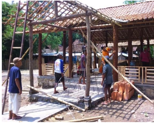
Figure 1. The Process of Building a Pavilion in Taman Jati Larangan Carried Out by The Local Community
