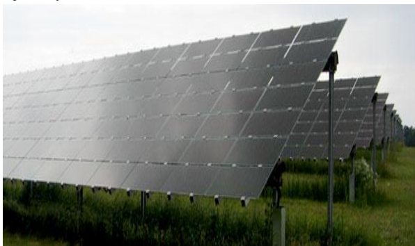
Fig.12- Solar panels installed at Village Nandha, Haryana at 30^\circ tilt angle
