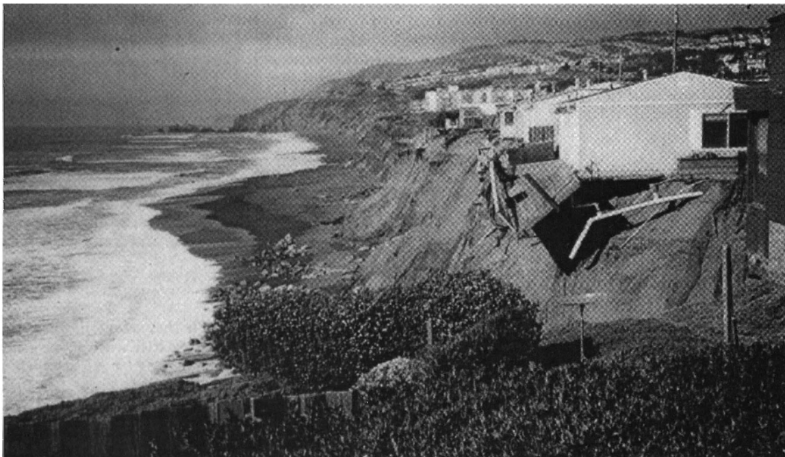
Figure 4. Erosion of the seacliff and undercutting of houses along the Esplanade at Pacifica in March of 1998. Rip-rap on the beach marks the location of the cliff toe before the winter storms. The scatter of these several-ton boulders testifies to the wave energies encountered along this section of the central coast during the 1997–98 ENSO storms. Photograph courtesy of Monty Hampton, U.S. Geological Survey.
