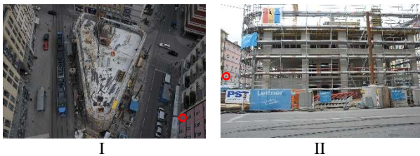
Figure 5. Example for two images taken on the construction site. Image I is taken from the crane. The red circles show a control point.
