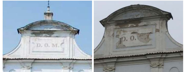
Figure 6. The upper part of the façade before (left) and after (right) the earthquake.
