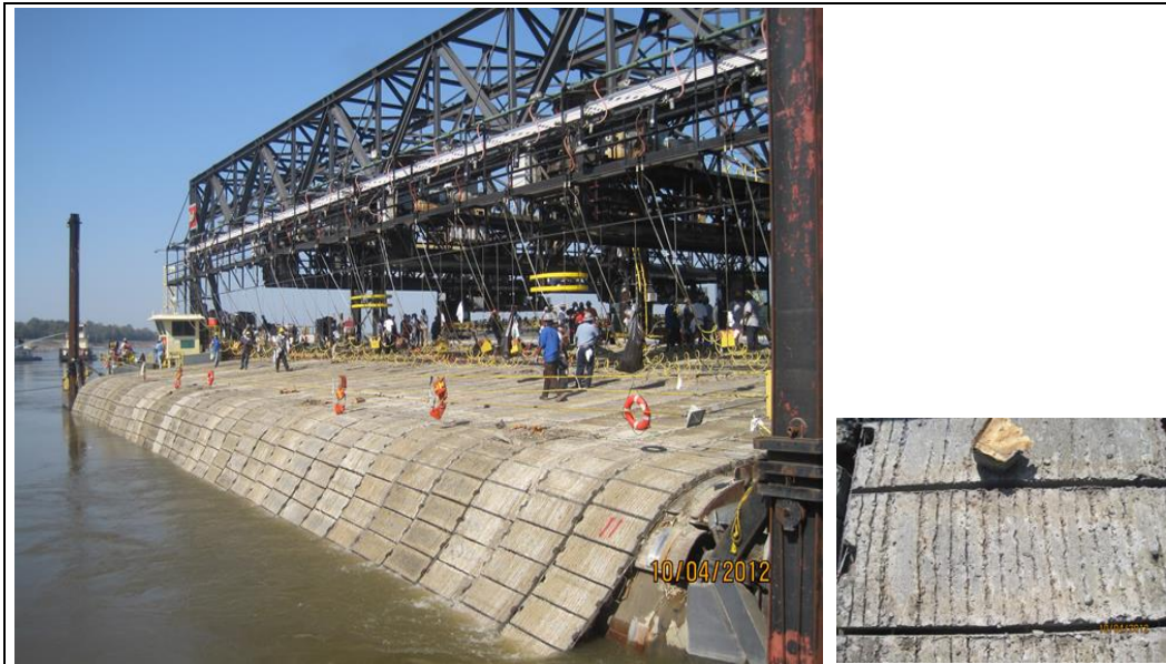
Figure 1. Mat Sinking Unit operating on the Mississippi River; inset of ACM grooves.
