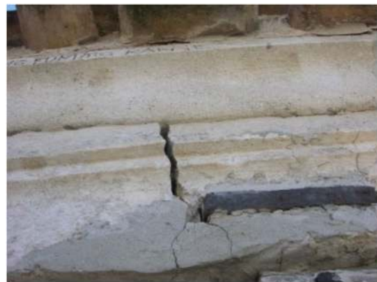
Vertical crack on the exterior top level of the façade
