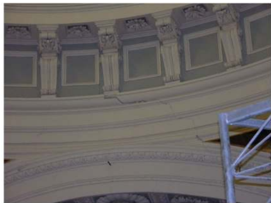
Diagonal crack on the north portion of the drum
