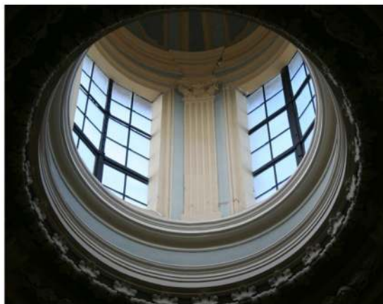
General view of the lantern with evident cracks at its base and top
