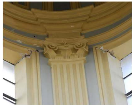
Detail of the horizontal crack at the top of the lantern
