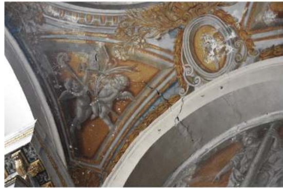
Crack on the abutment of the South-central vault of the chapel
