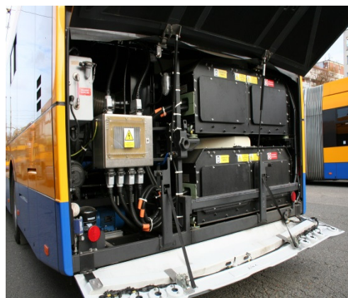
Fig. 2. Complete set of traction batteries nLTO mounted in vehicle
