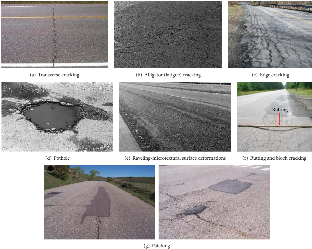
FIGURE 5: Photographs of typically observed road pavement distresses.
