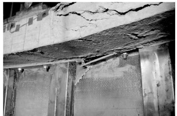
(b) Shear failure of FRP girder
