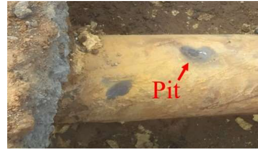
Fig. 14: The photo of found pit in pipeline.
