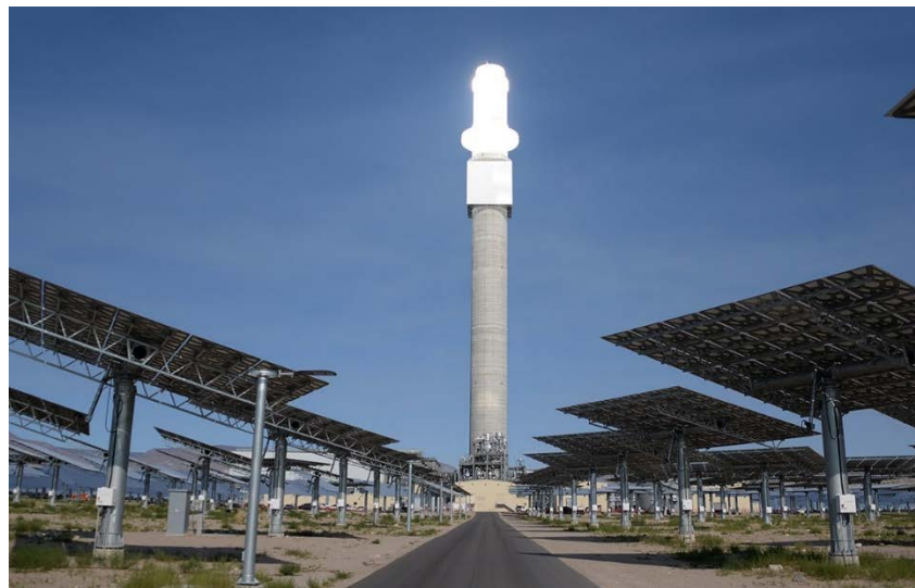
Figure 6-3. Crescent Dunes nitrate salt receiver Source: Google Images
