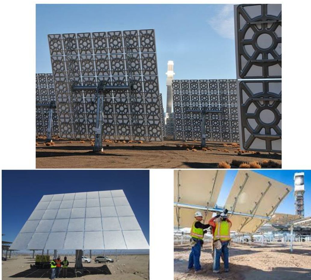
Figure 6-1. Both large and small heliostats are used in today's commercial power towers Source: Crescent Dunes (large) and Ivanpah (small)
