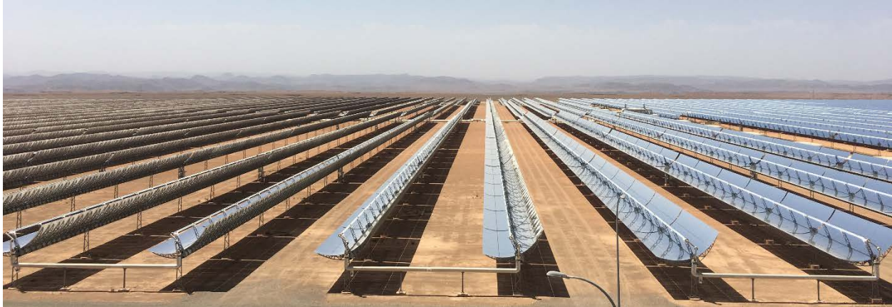
Figure 5-1. 160-MW e Noor Ouarzazate I Parabolic Trough Plant, Ouarzazate, Morocco
