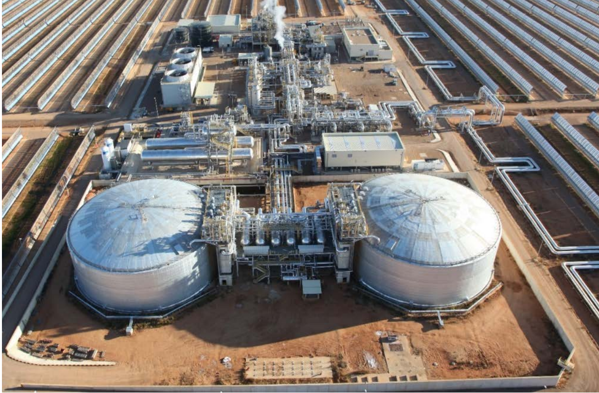
Figure 5-5. 50-MW Termosol 1 Plant with 9 hours of indirect molten-salt thermal energy storage (Spain)
